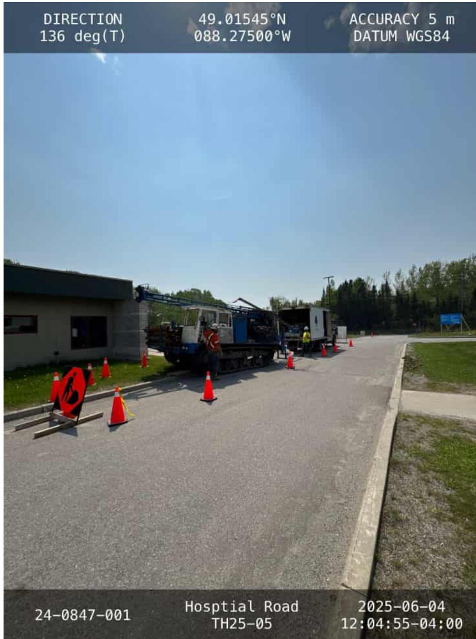
Photo 5: Drill Rig Setup at TH25-05 Located Near Southwest Corner Of Medical Centre Building, Looking South
