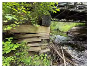
Figure 20: South Crib - Severe Rot
