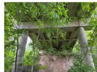
Figure 28: North Pier, South Side, Small Spill (Left)
