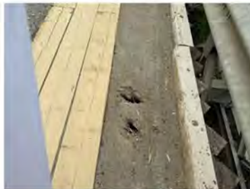
Figure 6: Deck Rot - NW
