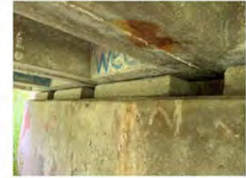
Figure 18: North End - Rust Staining and Delamination of Girders 4 and 5 From East.
