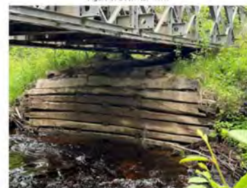
Figure 19: North Crib - Severe Rot.
