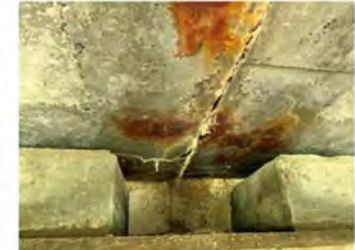
Figure 17: North End - Rust Staining and Delamination of Girders 3 and 4 From East.
