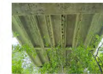
Figure 27: Underside of Structure at Midspan - Small Spills, Delaminations, Rust Staining.
