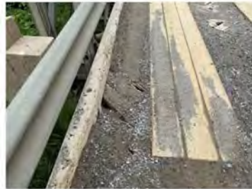
Figure 5: Deck Rot - SW
